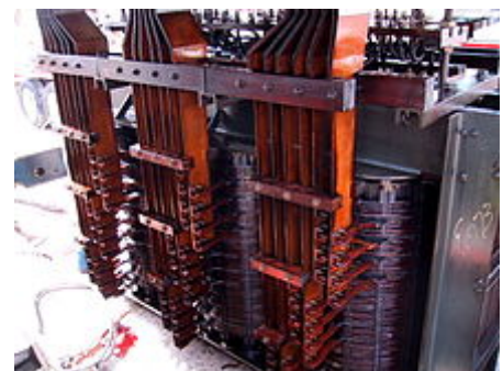
Heavy windings in an Electric Arc Furnace transformer.
