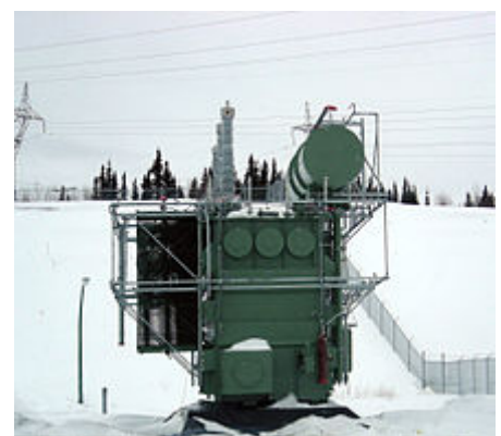
High voltage, three phase, oil-cooled transformer
